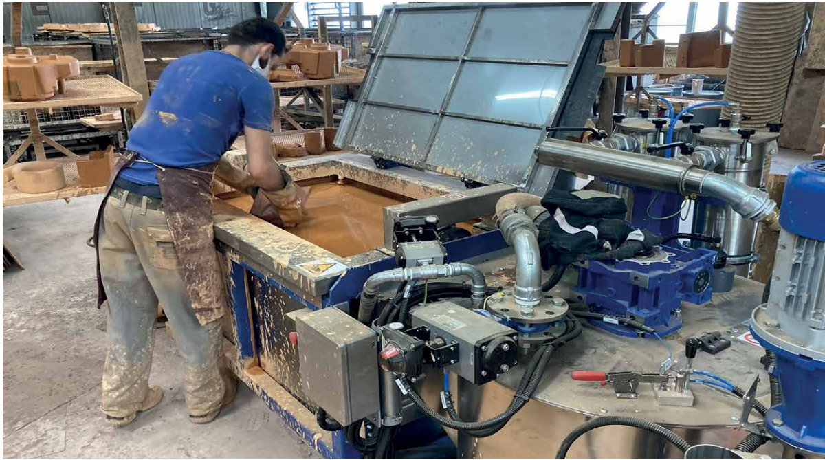
Another coating dip tank. In St. Leon-Rot the dip tanks are located on two floors, while in Elsterheide on one floor.
